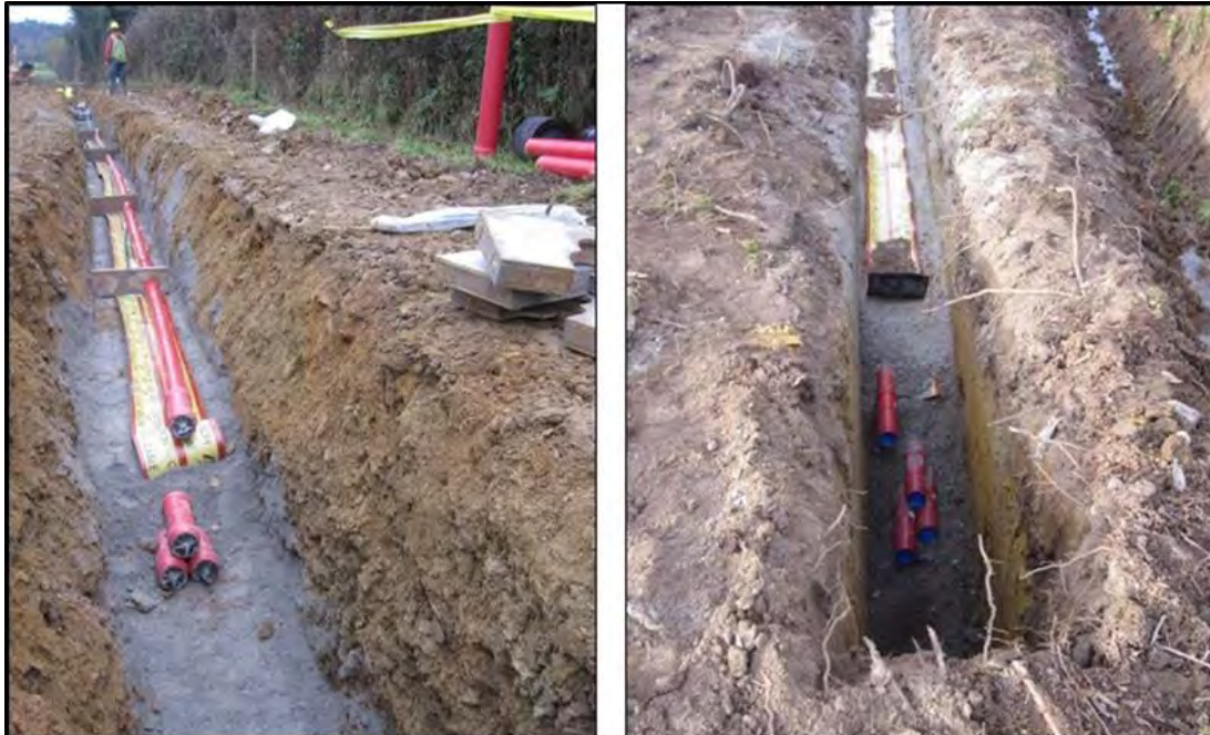
Plate 4-7 Typical Cable Trench View
