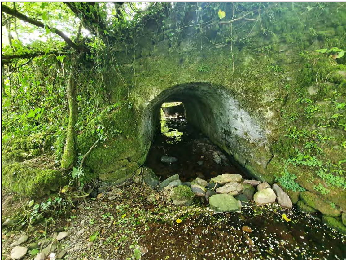
Plate 7-18 The Glennaglogh River, located along the turbine connector route, which will be located within the existing road over the bridge.
