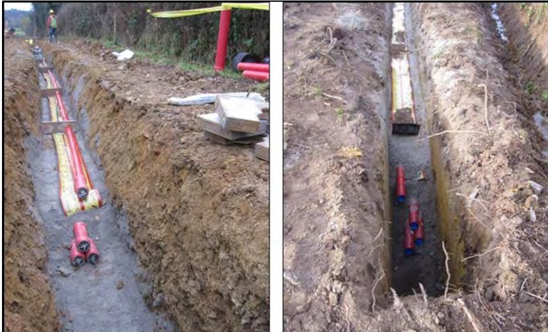
Plate 4-7 Typical Cable Trench View
