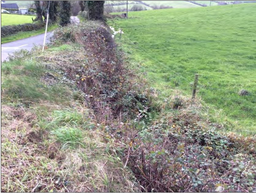
Plate 14.69: Section of road widening at Killea townland looking S (Lombard's Cross Roads)
